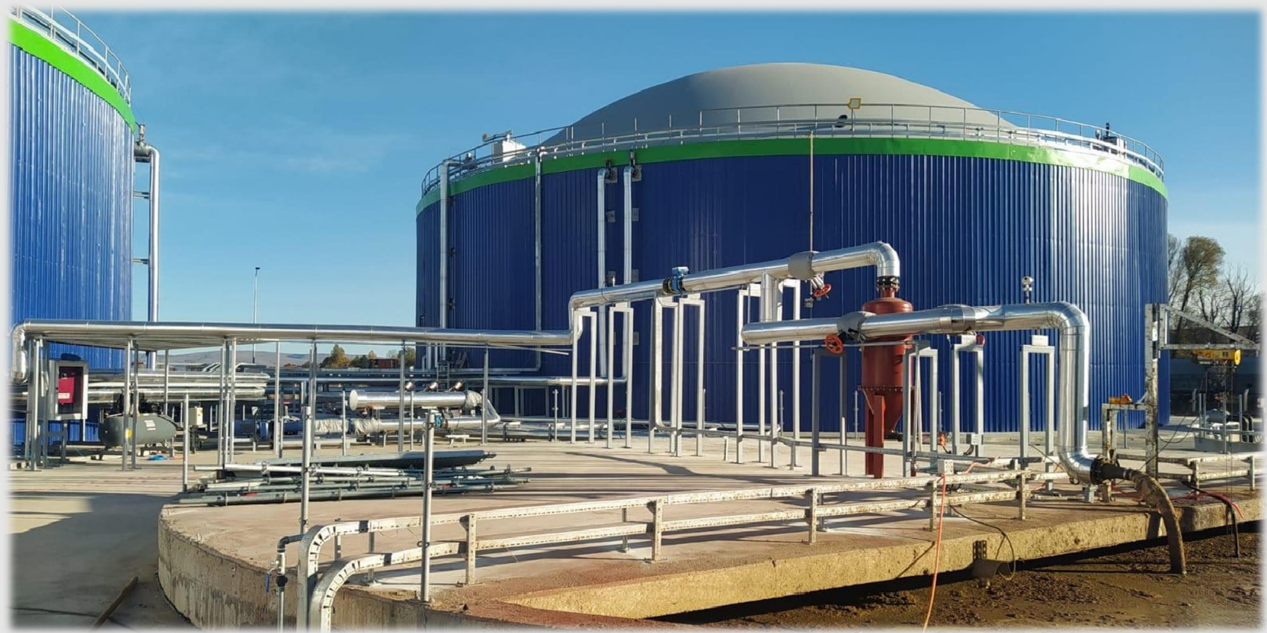
BIOGAS POWER PLANT / GAZIANTEP
